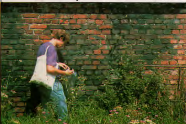
Illustration 10: The outside wall of the hydrocyanic acid delousing installation of building BW 5b is intensely blue in colour from the effects of hydrocyanic acid. With time, the cyanide penetrated the walls and reacted with iron to form the pigment, unaffected by 50 years of weathering.
