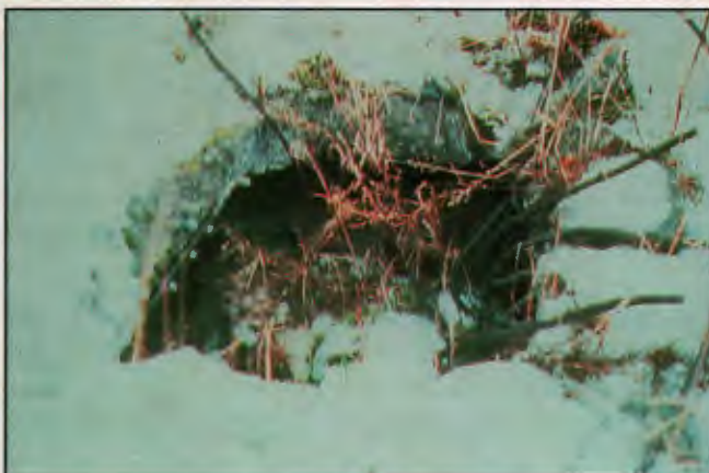
Illustration 6: Alleged Zyklon B vent in the roof of the morgue («gas chamber») of Crematorium II. The steel reinforcement rods in the concrete were never even removed. They were simply bent apart, and backwards.
